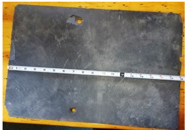
An original 12x18 inch slate shingle used on the roofs of the buildings built in 1881-1882.
